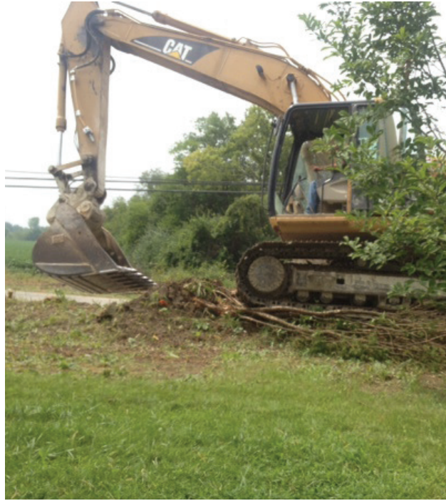
2) Heavy equipment tearing out the trees in front of the Granato home.
